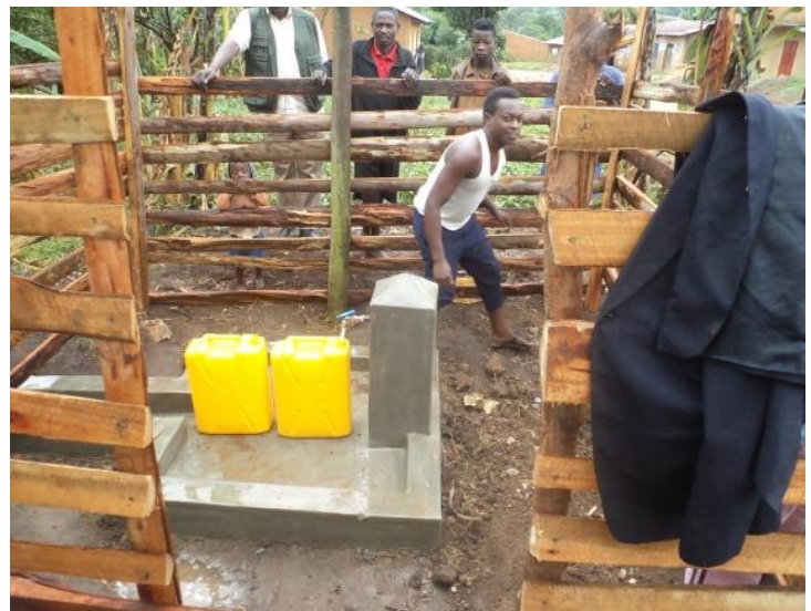
One of the finished and connected with water public tapstand
