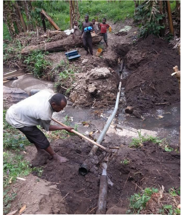
A stream crossing pipe that was washed away by floods at Karerema
