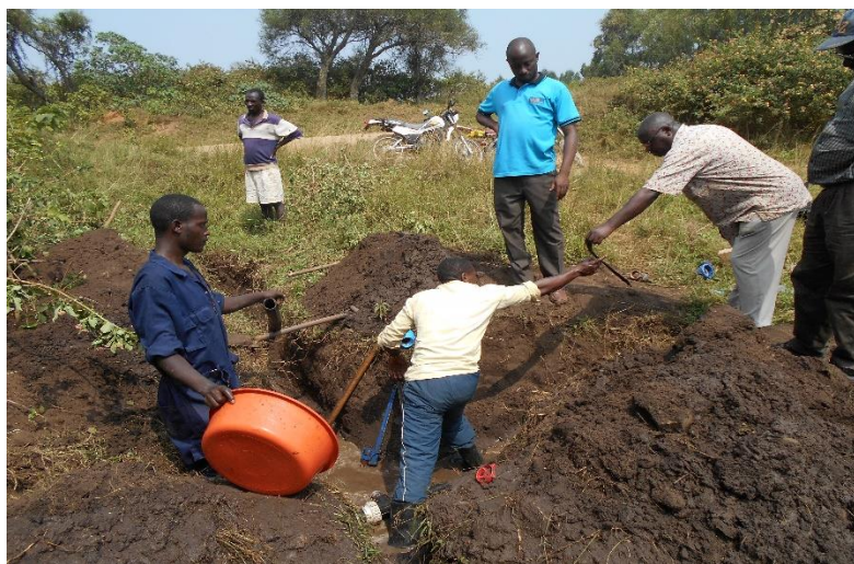
WatSan staff working with the community to replace a faulty control valve on Nyambizi GFS
