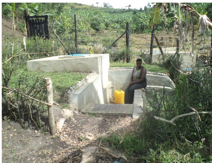
Low yield spring constructed adjacent to Kiringa GFS water source
