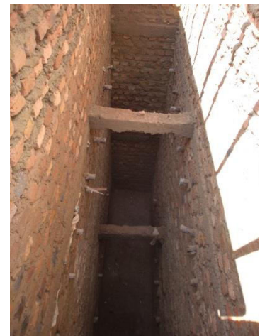
View inside lined pit showing full depth. Ring beams spanning width can be seen.
