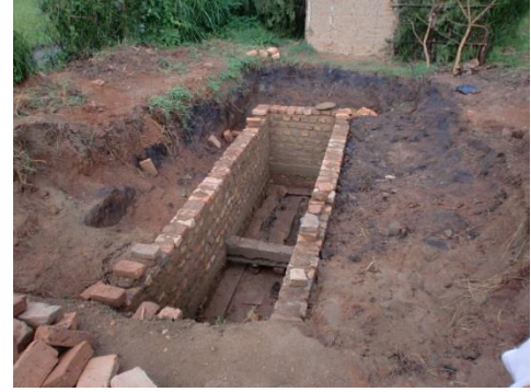
Pit latrine after construction of pit lining including ring beams (full depth not shown here)
