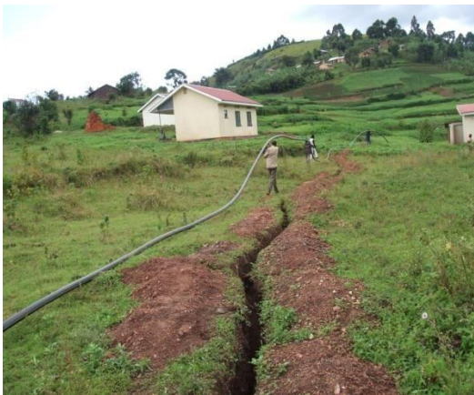
Laying of a pipeline at Kabuga HC II before the construction of a double tapstand at this centre
