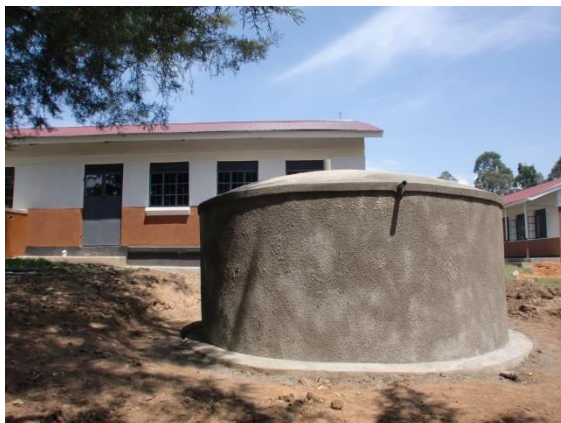
30m 3 RWH tank constructed as part of the 2 nd phase of the project
